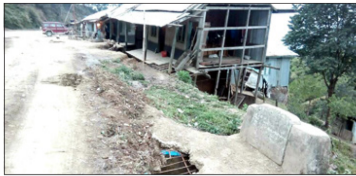
A view of the damaged house and sunken road in Khaivarentang village
